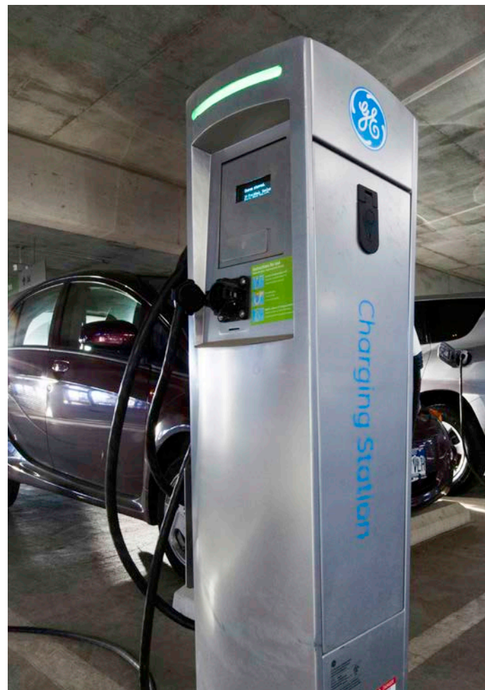
Photo by Dennis Schroeder, NREL 24540
