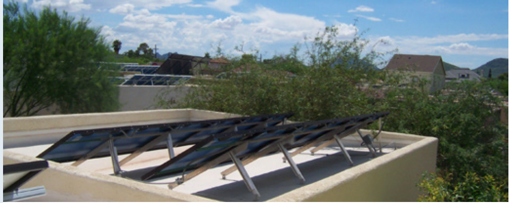
Solar photovoltaic and water heating panels are mounted on the flat roofs.
