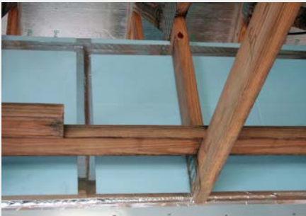
Completed chase ready for insulation wrap and drywall. Note sealed bottom using ½-in blueboard.
