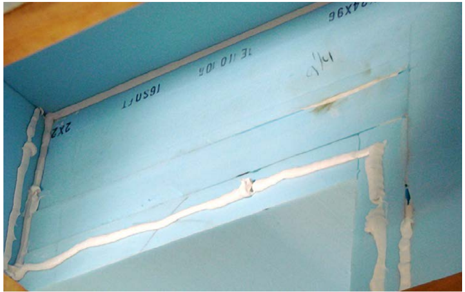
Ready to install the second layer of blueboard. Note the staggered joints and adhesive used to seal seams and attach layers together.
