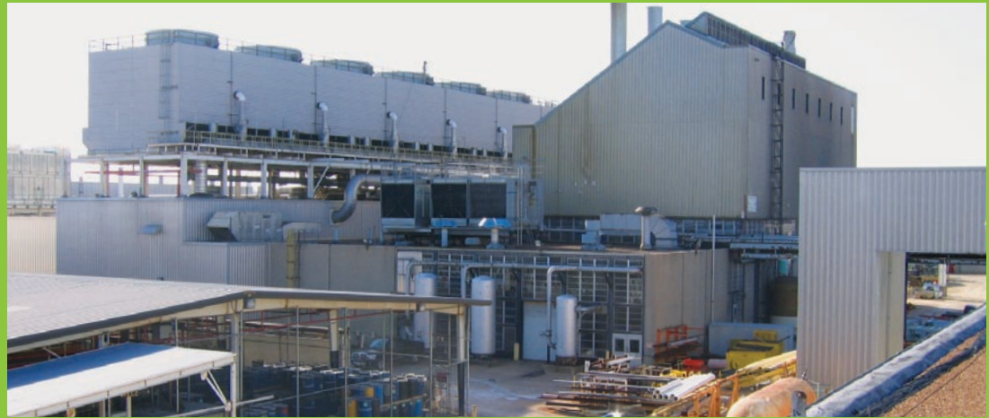
The powerhouse at Chrysler's St. Louis Assembly Complex provides steam, chilled water, and compressed air to both the north and south plants.
