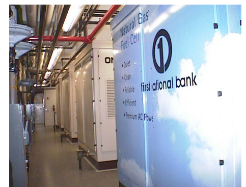
Fuel cells (right) and gas regulators (left) installed at the First National Technology Center.
