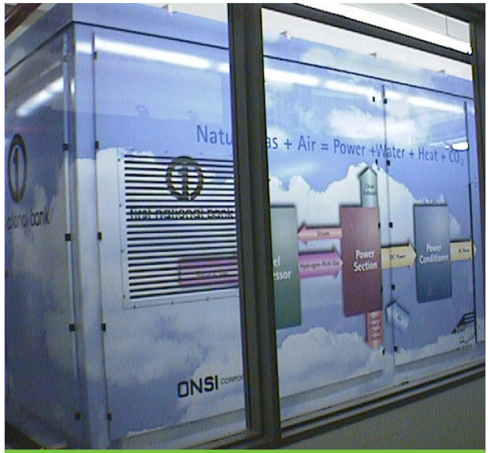
UTC Power PC25C fuel cells installed in the basement of First National Bank of Omaha’s Technology Center in Omaha, Nebraska.
