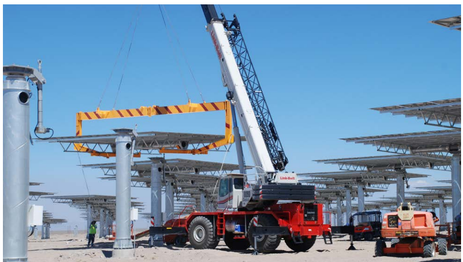
During construction of Crescent Dunes , 600 jobs were created. Photo Credit: SolarReserve, LLC
