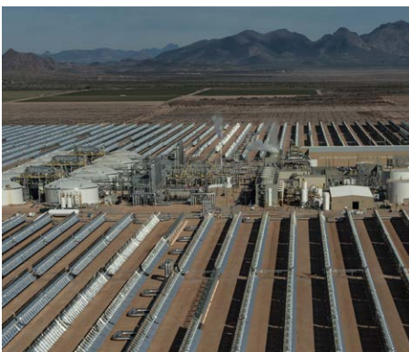
Solana, Photo Credit: Abengoa Solar, Inc.
