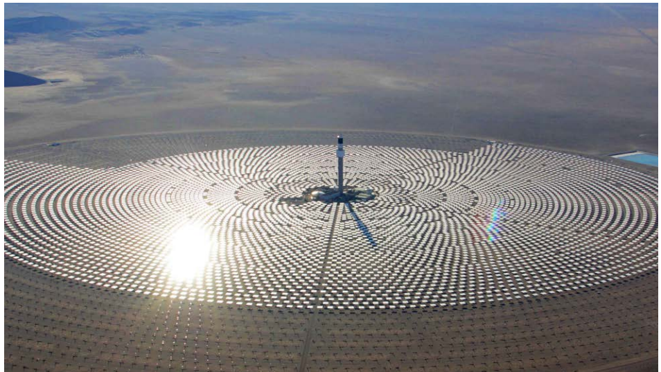
Crescent Dunes is the largest power plant of its kind in the world. Photo Credit: SolarReserve, LLC
