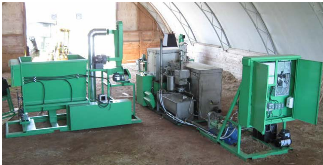
CanmetENERGY Auger Pyrolysis System
