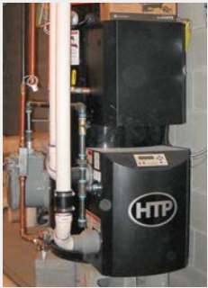
House #2: high-mass, modulating, condensing water heater; variable-speed pumps; baseboard convectors; no primary-secondary piping
