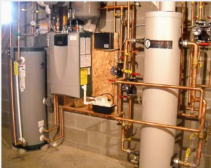
House #3: low-mass, modulating condensing boiler; indirect domestic hot water tank; variable-speed pumps; baseboard convectors. A buffer tank was compared to primary-secondary piping. Constant temperature operation was compared to thermostat setback.
