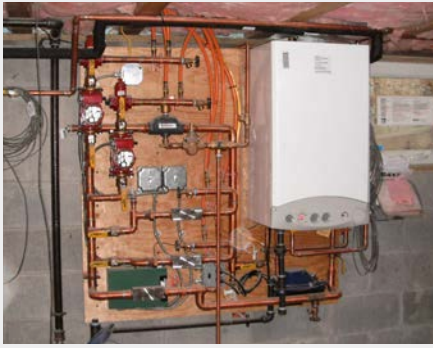
House #1: modulating condensing boiler with an integral tankless coil for domestic hot water and under floor radiant tubing
