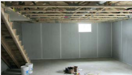
Exposed polyisocyanurate insulation panels in basement provide R-13 insulation and a finished appearance. All floor framing is open-web trusses to accommodate mechanicals.
