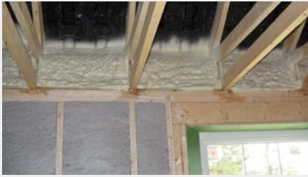
Ten-and-a-half inches of dense-pack cellulose in double 2x4 walls, raised heel trusses, and foamed-in plastic rafter vent baffles.
