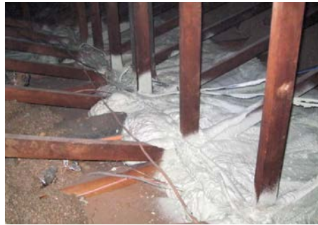
Application of membrane and spray foam to seal ductwork and air leakage pathway
