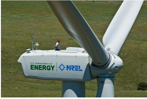
DOE 1.5MW research wind turbine installed at the National Wind Technology Center (NWTCC) in Colorado
