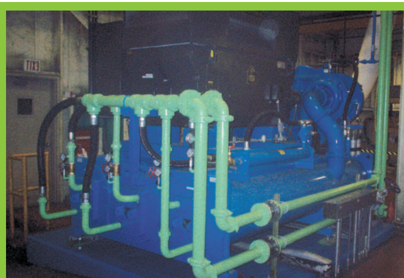
The Santa Clara plant used rebates from Silicon Valley Power to replace an aging compressor and achieve annual compressed air energy cost savings of approximately $120,000.
