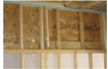
(top) Holes for electrical boxes and wiring and plumbing pipes were sealed with spray foam. Seams at corner framing and bottom plates were caulked.
