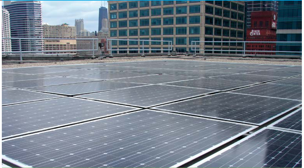
Photovoltaics installed on the Harold Washington Social Security Center in Illinois as part of an ESPC. Photo from U.S. Social Security Administration, NREL/PIX 19006
