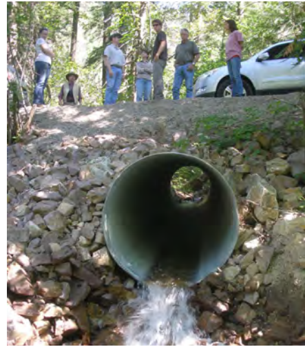
A BPA mitigation monitoring team inspects a new culvert installed to prevent vehicles from driving through a stream at the Libby-Troy Rebuild Project in Montana.
