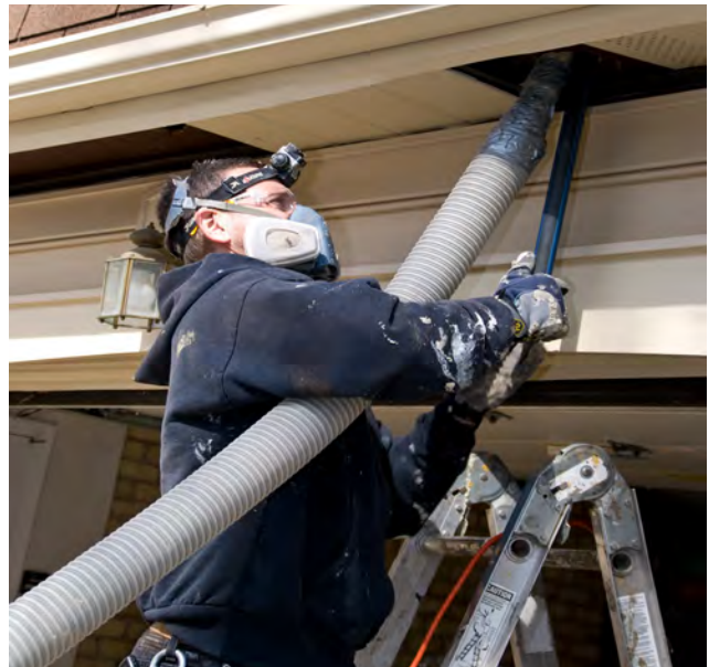
Improving insulation normally would be exempt from Section 106 review under the programmatic agreement. (photo: SMS)
