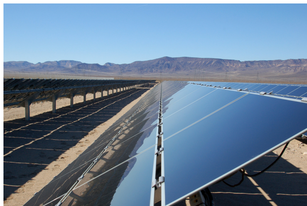
Arrays of ground-mounted PV modules would be manufactured and installed at Topaz Solar Farm by the project proponent, First Solar, LLC.
