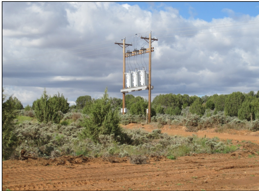
Figure 3-13. Transformer Substation on Old Landfill Road adjacent to Proposed Pilot Plant Site
