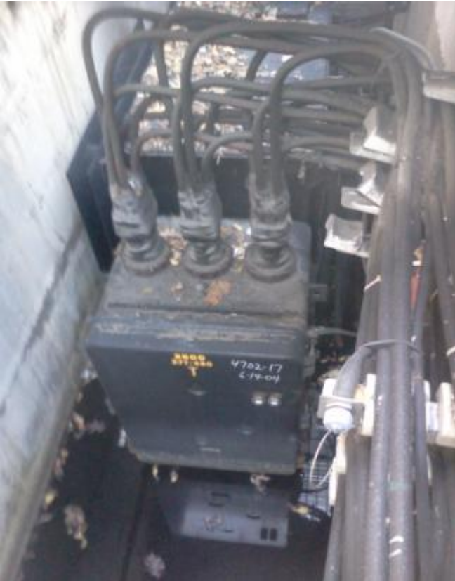
Typical Network transformer in a vault
