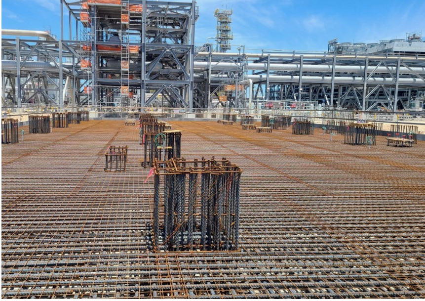
Photo 5: End Flash Gas Foundation
