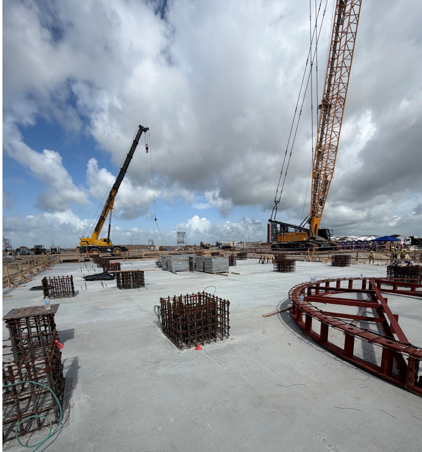
Photo 5: End Flash Gas Foundation
