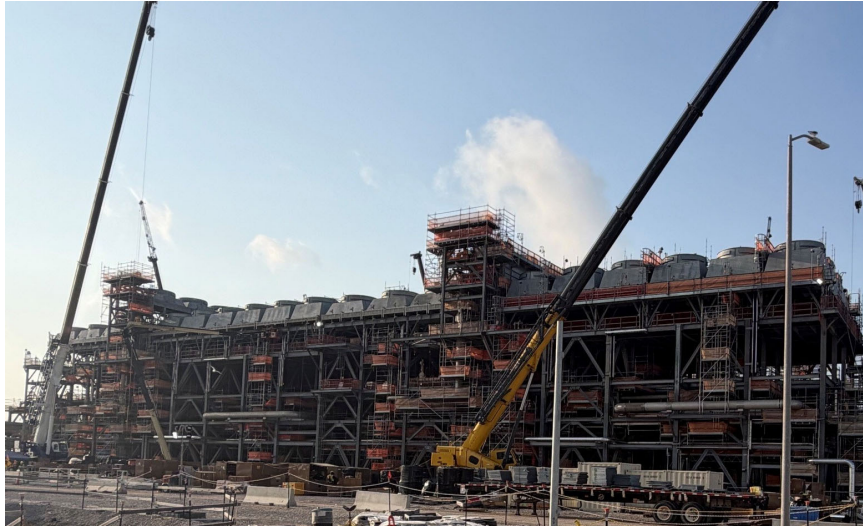
Photo 1: Train 7 Cryogenic Rack Area
