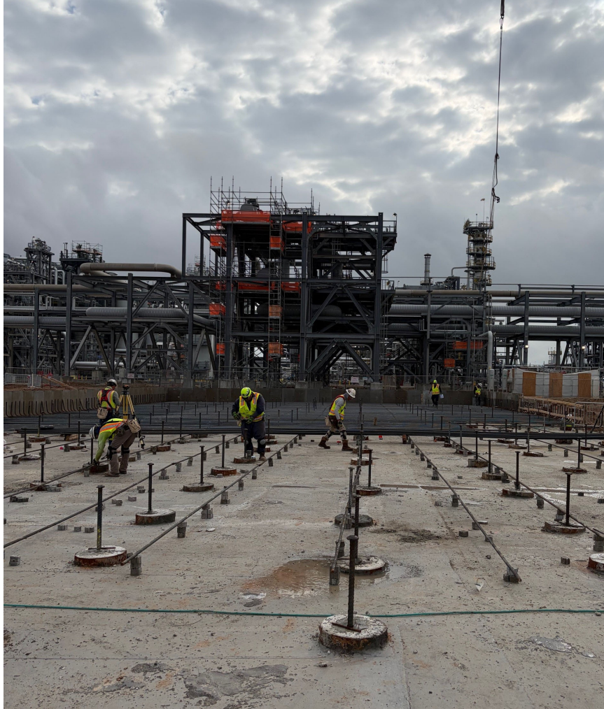
Photo 5: End Flash Gas Foundation
