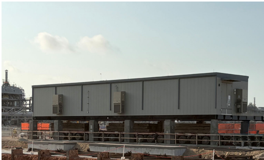
Photo 4: Train 9 Utility Substation
