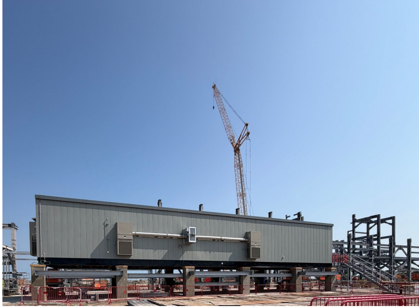
Photo 3: Train 8 Utility Substation
