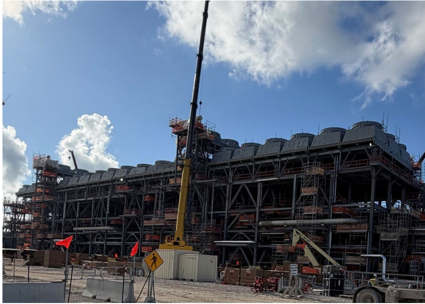
Photo 1: Train 7 Cryogenic Rack Area
