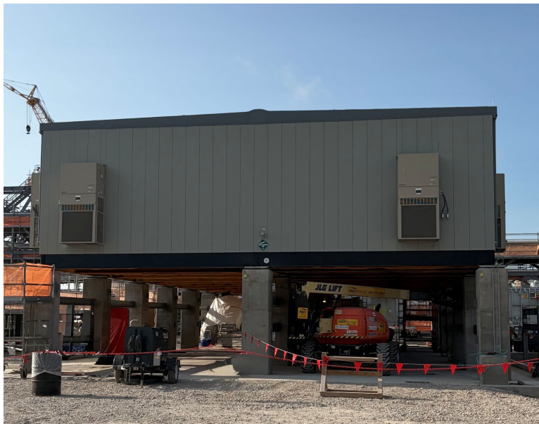
Photo 2: Train 8 Liquefaction Substation
