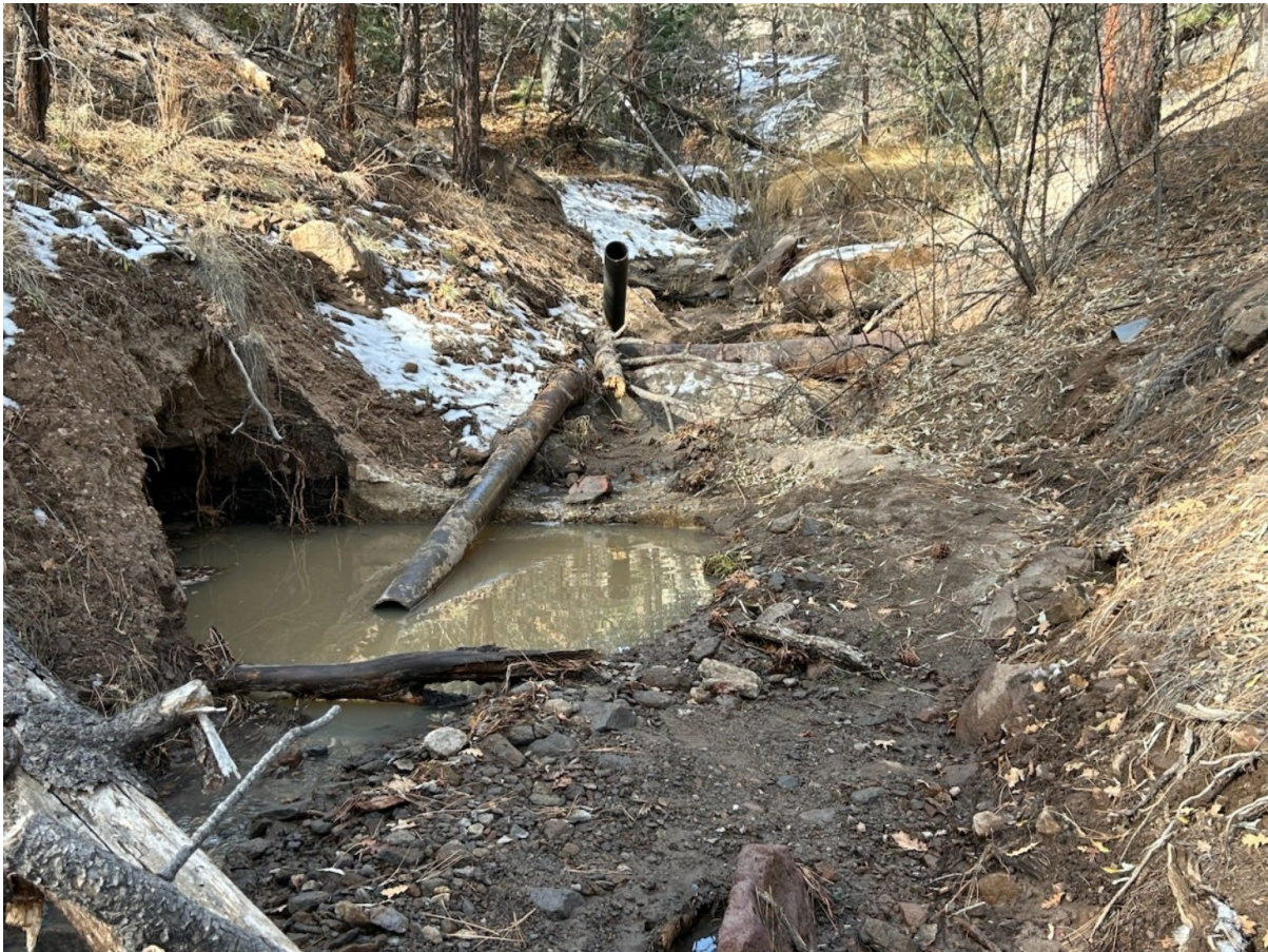
Photograph 9. View upstream at the canyon-bottom repair area and approximate location of the failed 18-inch transmission main. Late February 2026. Photograph 9 shows the constrained canyon-bottom work area and the approximate location of the failed transmission main.
