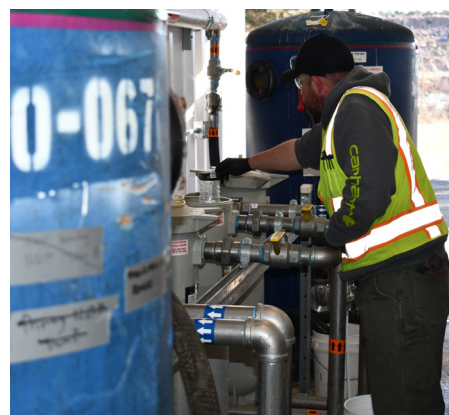
Ion exchange treatment system in Mortandad Canyon
