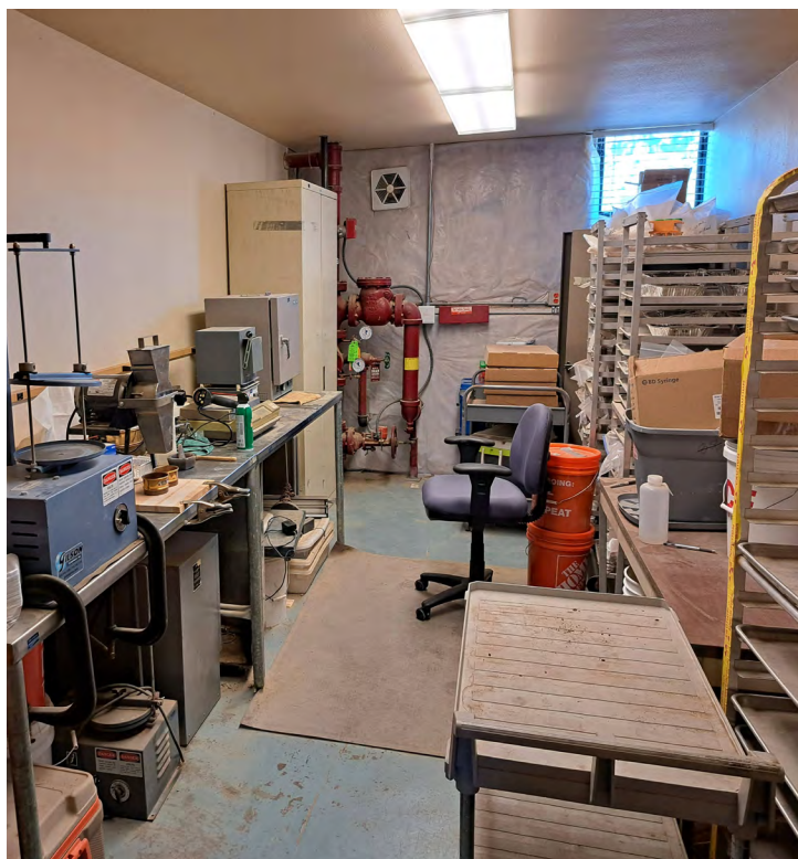
Solids processing room.
