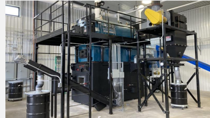
Fond du Lac Band of Lake Superior Chippewa (MN) Biomass District Heating System for its Brookston Community Center in 2025 Photo by Josh Gregory, DOE
