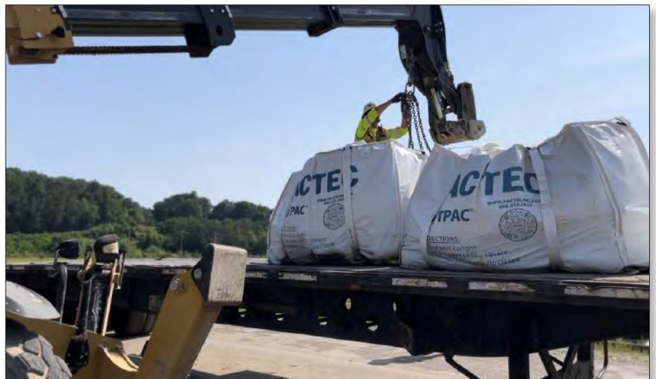
Workers supporting construction of Kairos Power's low-power demonstration reactor at the East Tennessee Technology Park load sacks of lead and copper from excavations for recycling, which will generate savings for the company.
