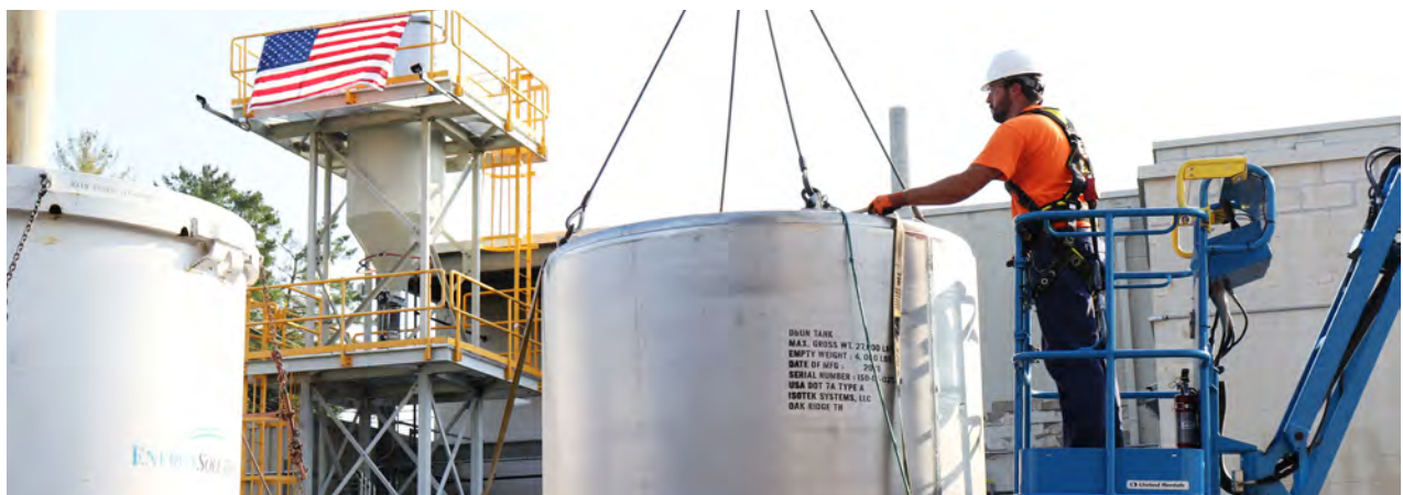
Processed U-233 is loaded for shipment and disposal
