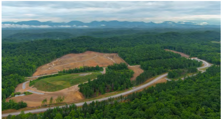
Early site prep is complete, and the future footprint of EMDF is taking shape
