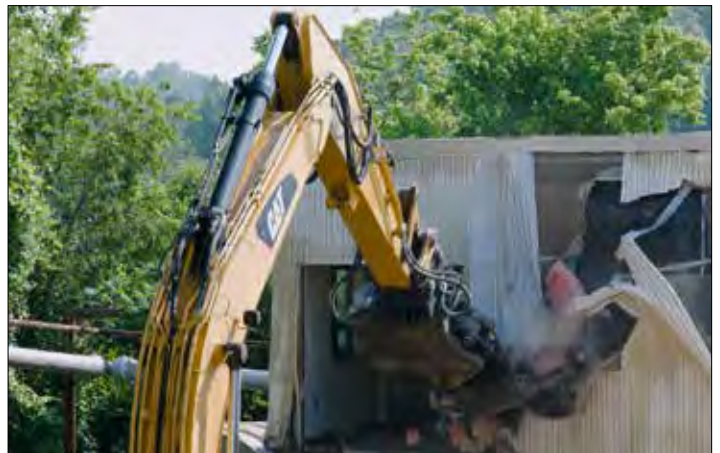
Demolition crews take the "first bites" of Building 3003 at Oak Ridge National Laboratory.
