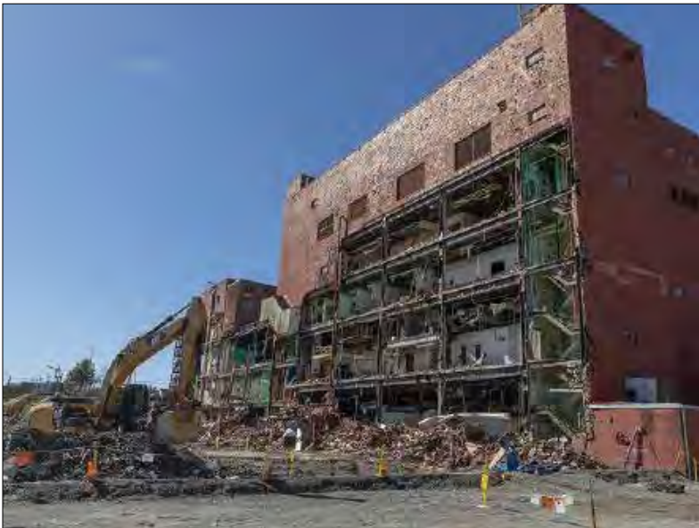
A view of demolition beginning on the six-story, 255,000-square-foot Building 9207, the final building in the former Biology Complex at Oak Ridge, which was demolished in 2021.
