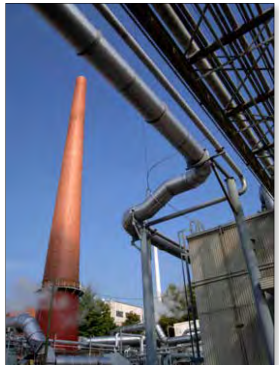
ORNL's Central Stack is part of an aging ventilation system that has reached the end of its usefulness.
