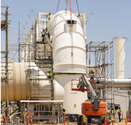
Underground Ventilation System (UVS)
