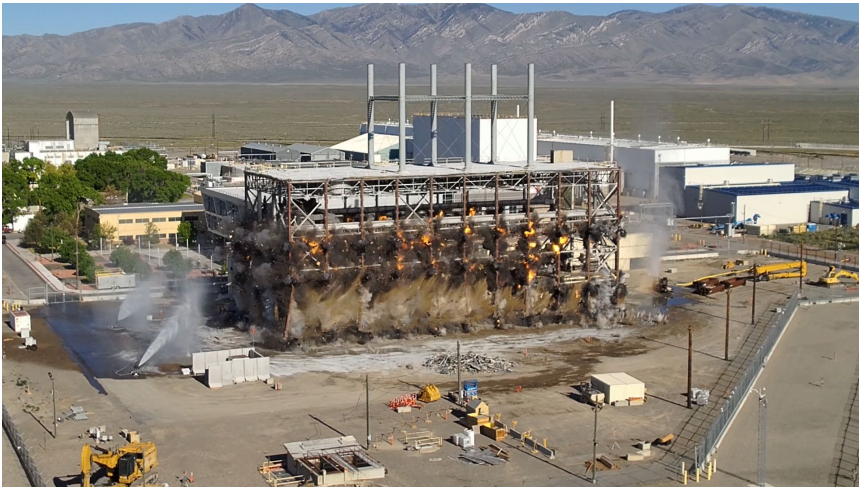
Energized demolition of the Navy's S1W reactor prototype building, reducing the long-term environmental liability and footprint at the site. (VIDEO)
