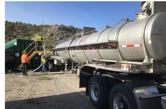
EM crews at Los Alamos National Laboratory empty purged well water into a truck for offsite disposal
