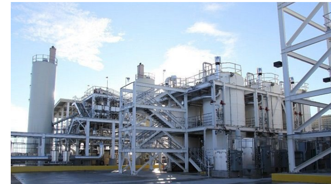
The 200 West Pump and Treat Facility, Hanford's largest groundwater treatment plant
