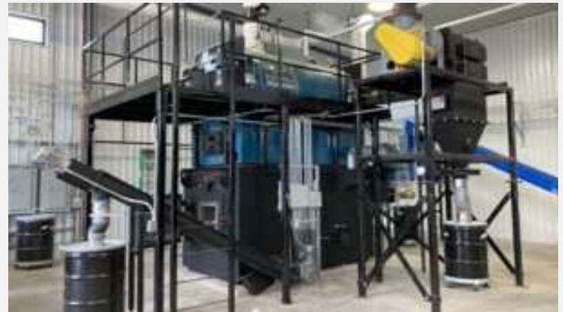
Fond du Lac Band of Lake Superior Chippewa Biomass District Heating System (Minnesota) installed a biomass district heating system for its Brookston Community Center, adding 3 MMBtu per hour of energy/ heating capacity. The system is projected to save approximately $31,000 annually. They celebrated with a ribbon cutting in June 2025. Photo by Josh Gregory / DOE
