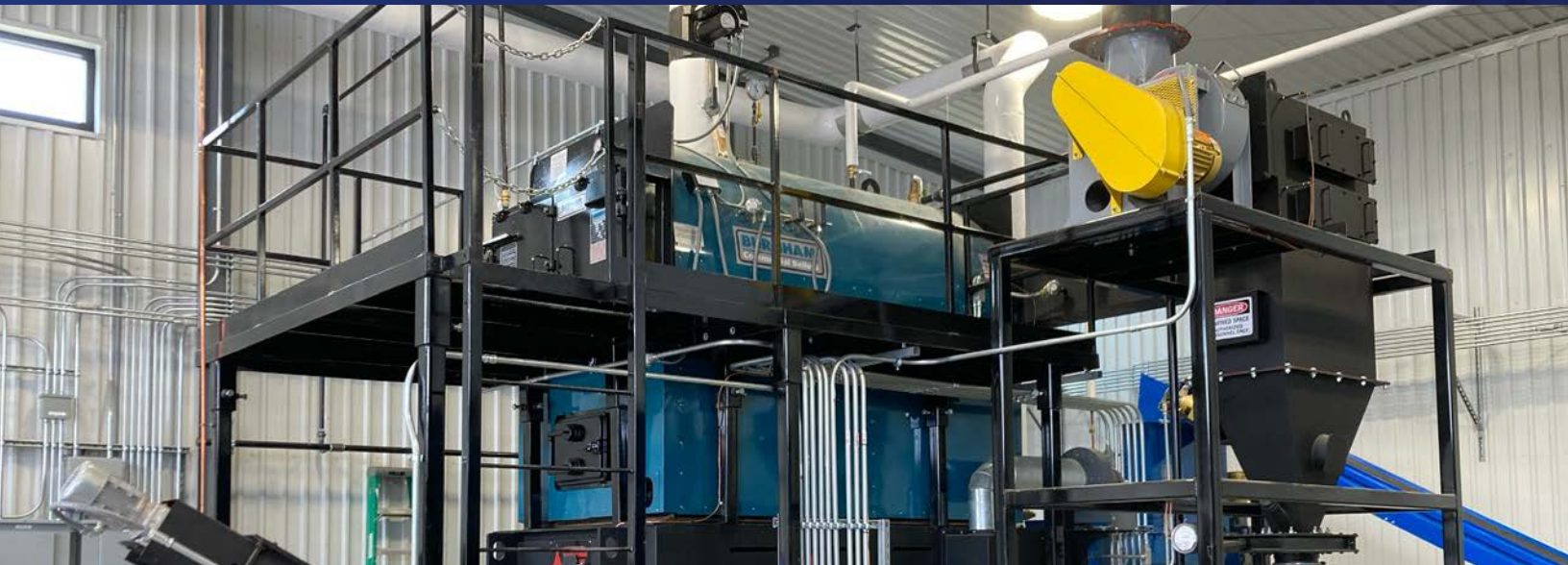
Brookston Community Center's woodchip-fueled hydronic boiler uses cutting-edge top-feed fuel technology to eliminate clogs and minimize maintenance downtime. Photo by Joshua Gregory, Office of Indian Energy.
