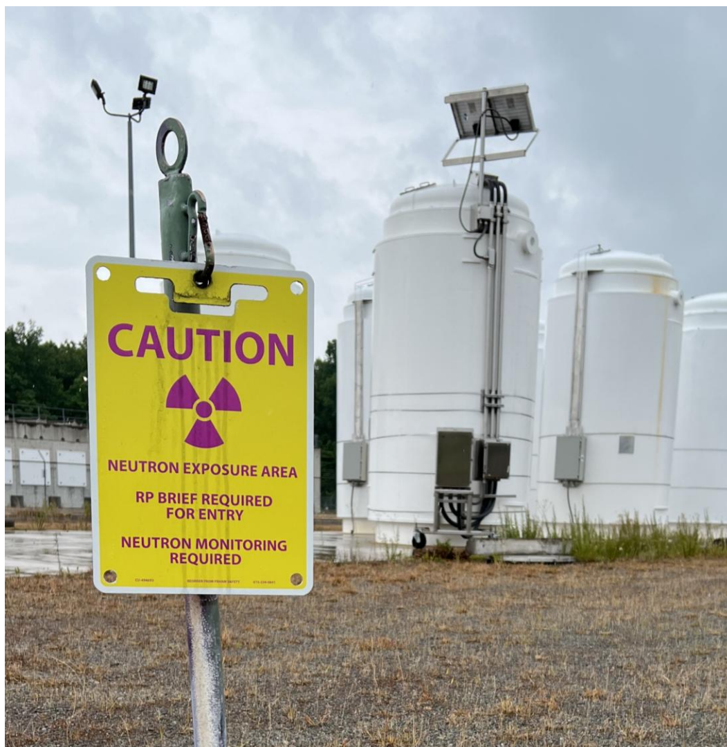
Figure 1-1. TN-32 storage casks at the North Anna Power Station site independent spent fuel storage installation (showing the TN-32B HBURC with solar panel).
