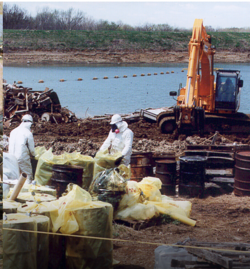
Barrels at the Weldon Spring Site, Missouri, raffinate pits required extensive cleanup during the Weldon Spring Site Remedial Action Project from 1987-2001.
