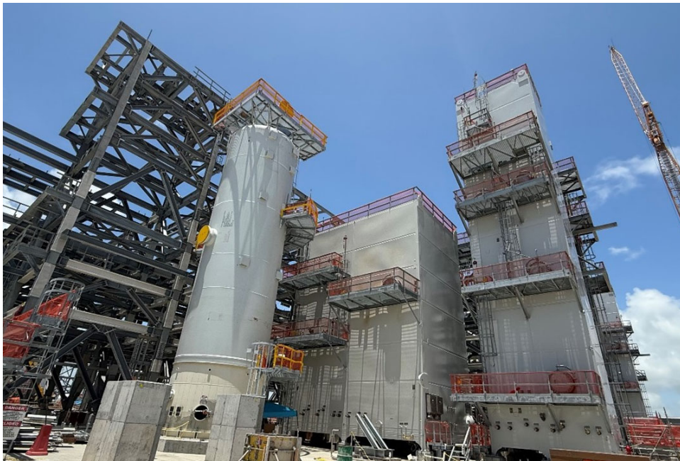
Photo 4: Train 6 Mixed Refrigerant Suction Drum and Cold Boxes
