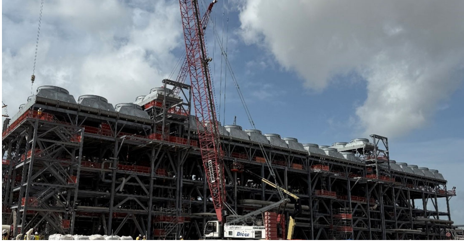
Photo 1: Train 5 Cryogenic Rack Area
