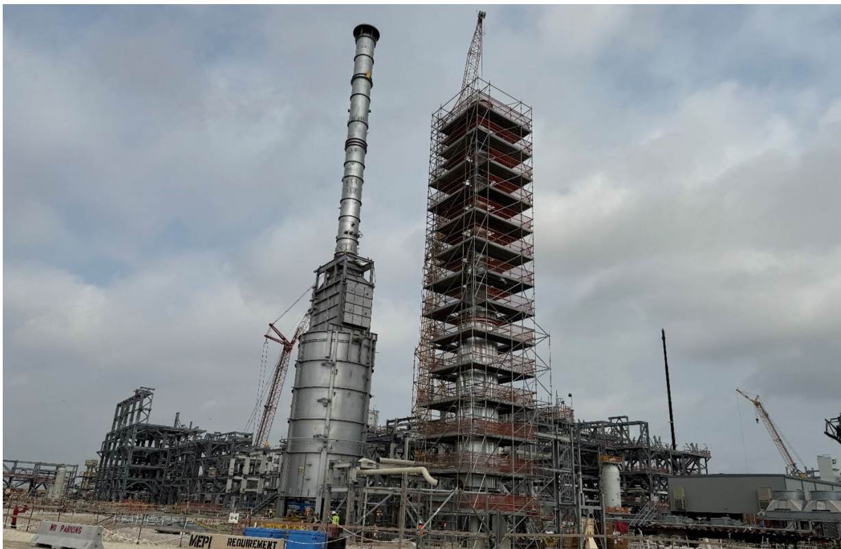
Photo 4: Train 6 Hot Oil Furnace
