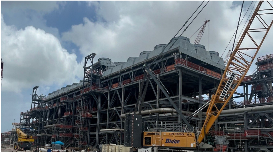
Photo 2: Train 5 Cryogenic Rack Area
