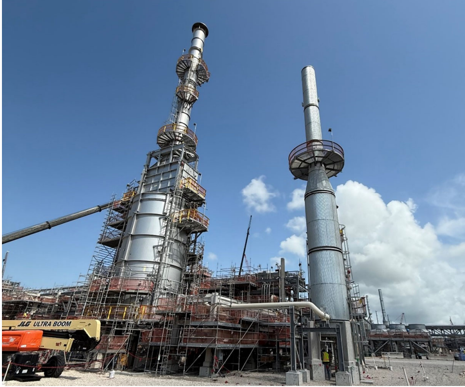
Photo 1: Train 3 Hot Oil Furnace
