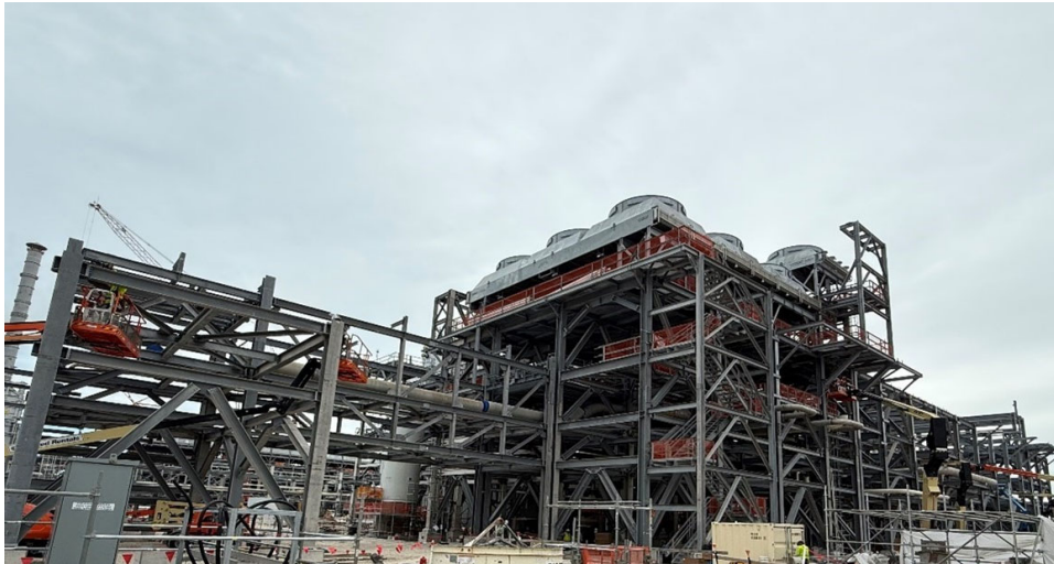
Photo 2: Train 6 Cryogenic Rack Area
