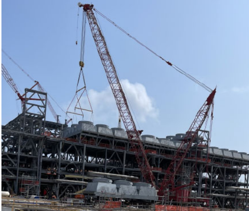
Photo 3: Train 5 Cooler Fans Setting
