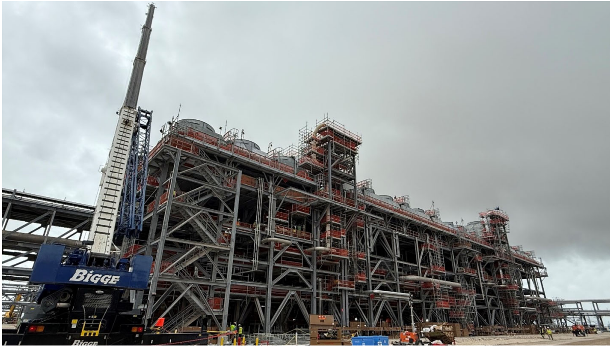
Photo 1: Train 2 Cryogenic Rack
