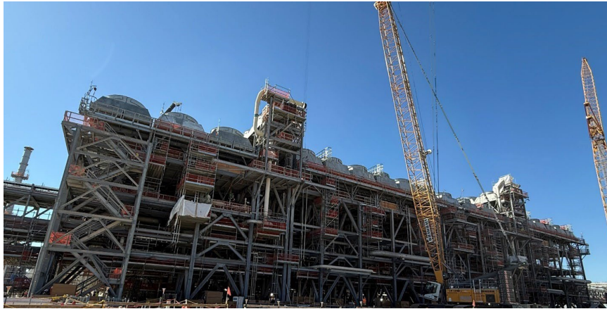
Photo 1: Train 2 Cryogenic Rack
