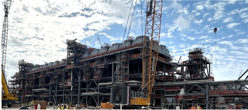
Photo 1: Train 3 Cryogenic Rack
