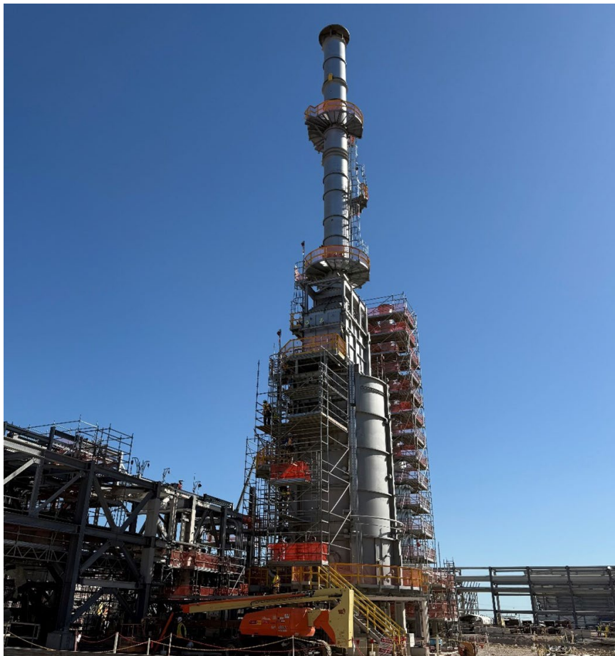
Photo 2: Train 3 Hot Oil Furnace
