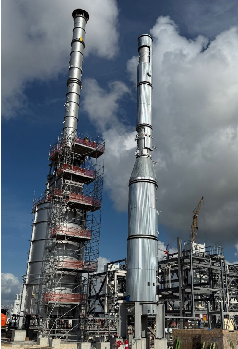
Photo 5: Train 7 Hot Oil Furnace
