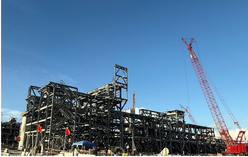
Photo 3: Train 7 Cryogenic Rack Area
