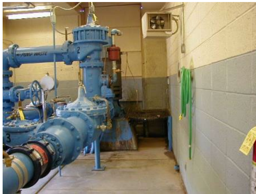
View inside of pump house at production well Buckman 1
