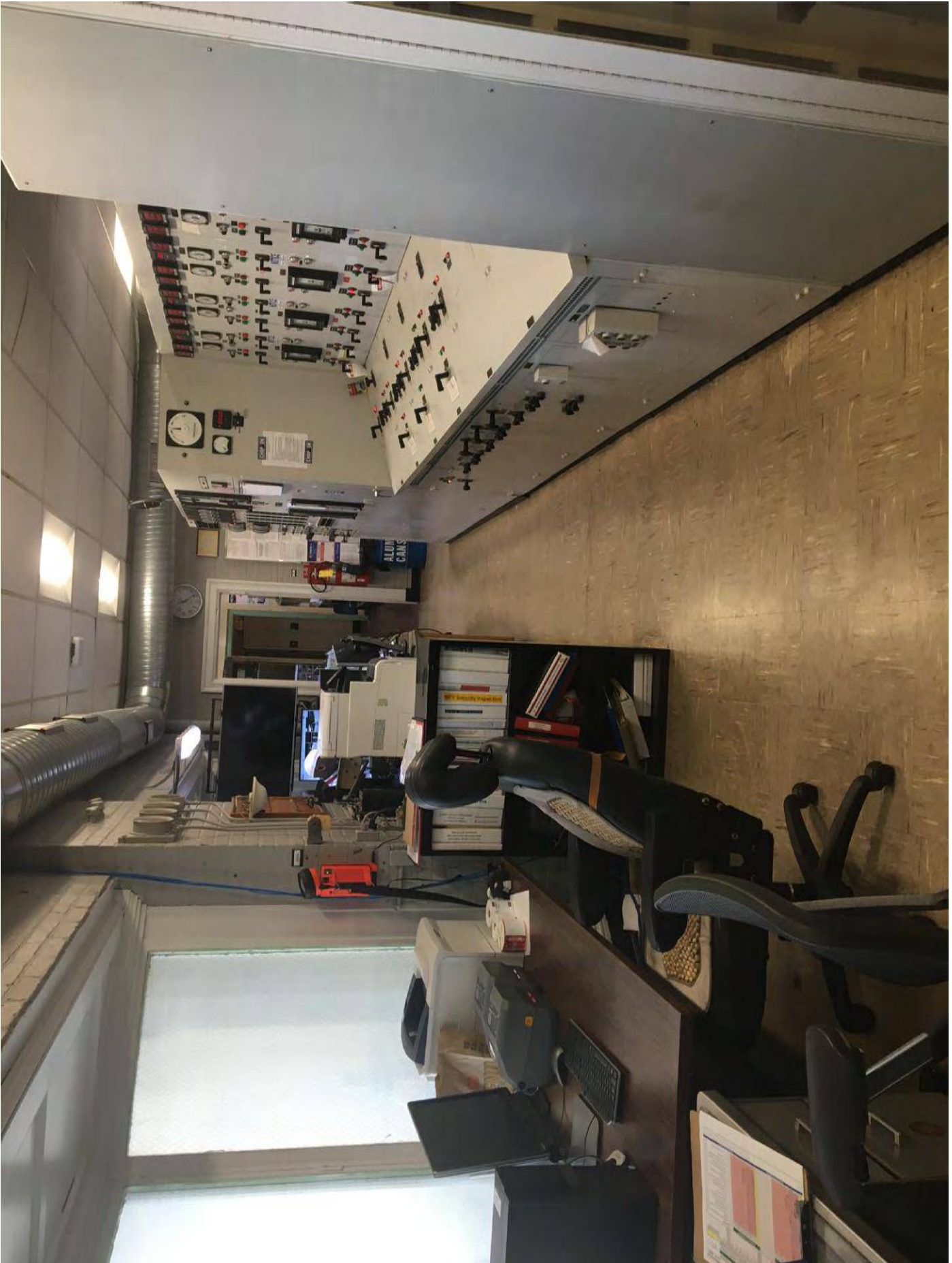
Figure 16. View of current control room.
