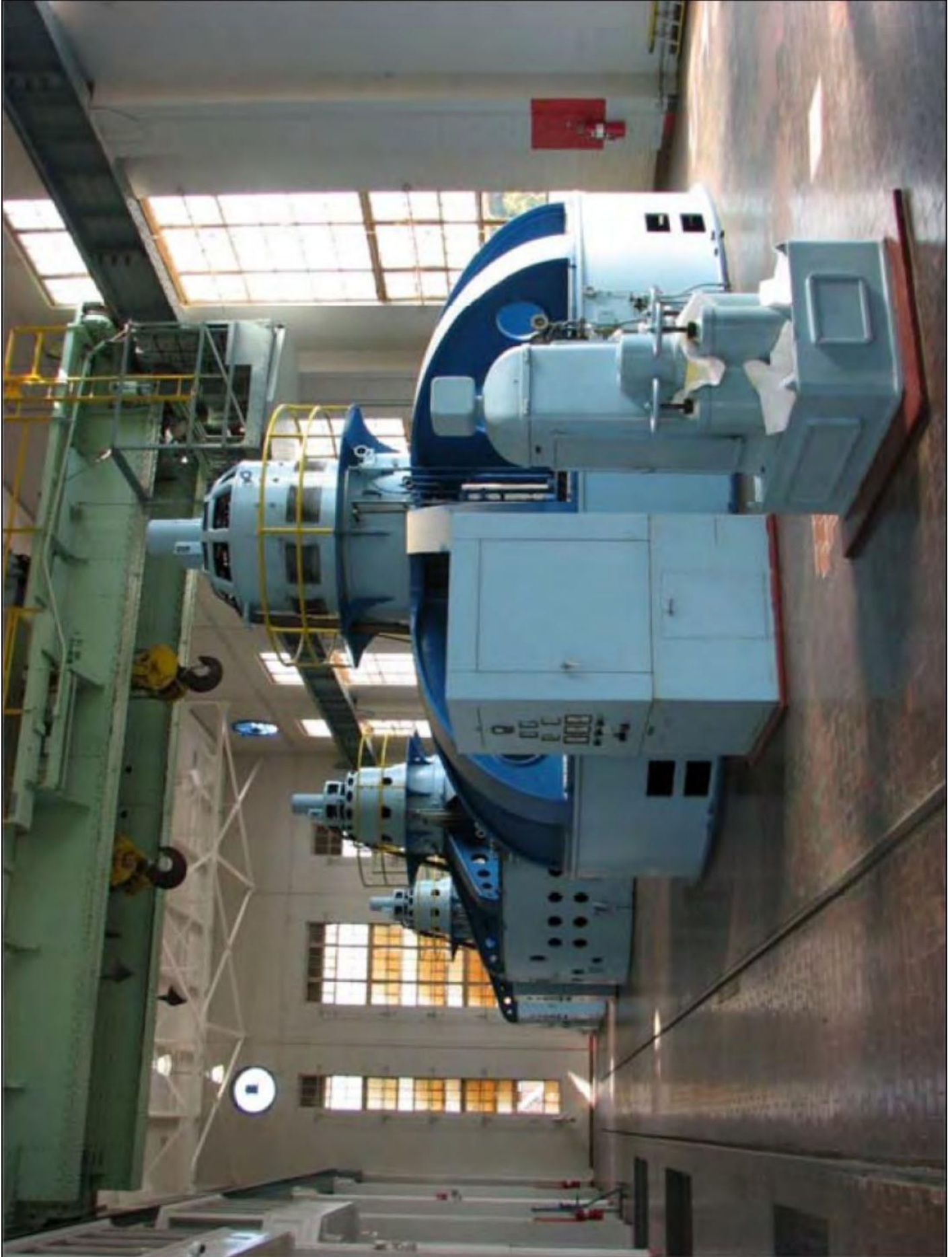
Figure 10. Photograph of generator floor.
