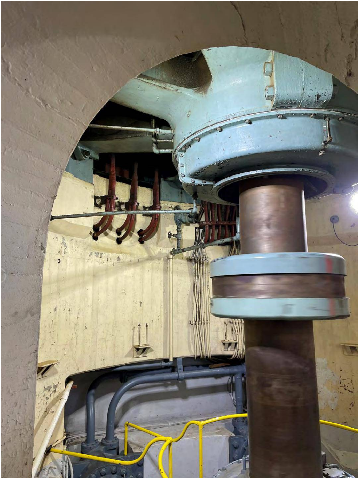
Figure 5. Photograph showing turbine detail.
