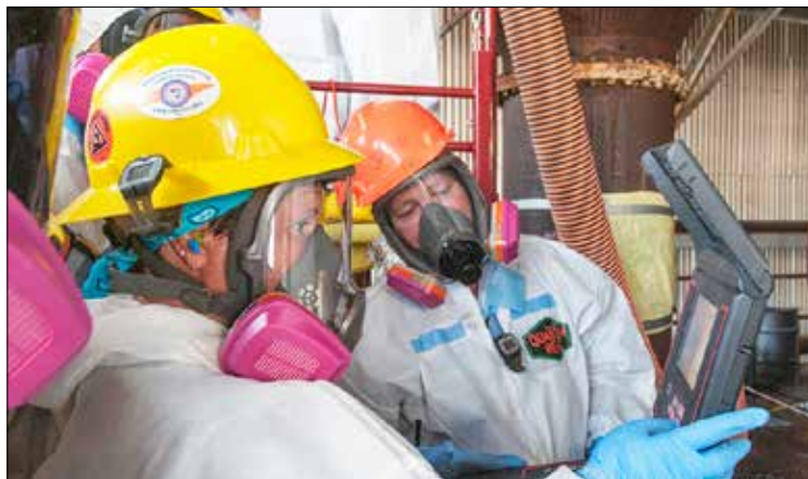
Oak Ridge workers address mercury contamination outside the Alpha-4 building at the Y-12 National Security Complex.
