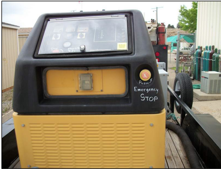
Figure 5. Emergency Stop Button
