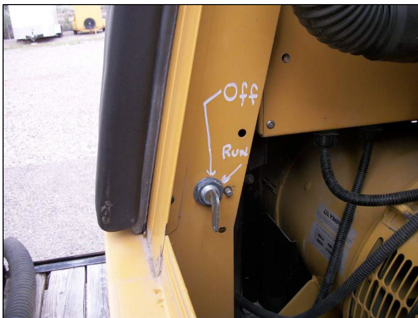
Figure 2. Battery Isolation Switch
