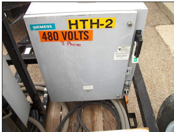
Figure 4. Typical Disconnect Switch
