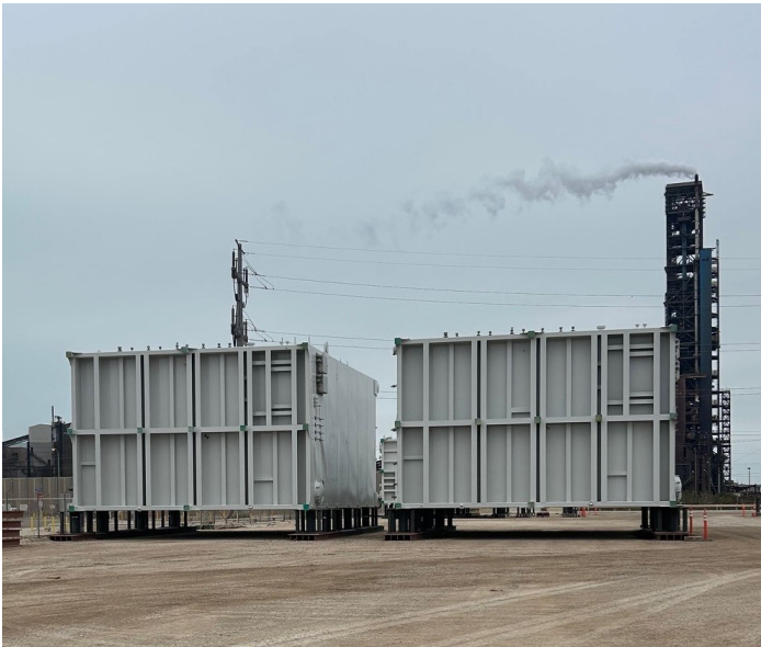
Photo 4: Train 7 Cold Boxes
