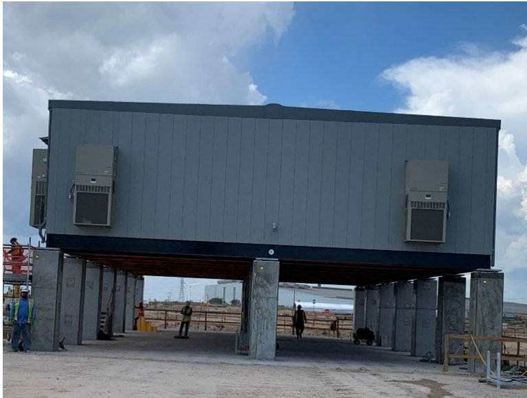
Photo 5: Train 7 Liquefaction Substation Set
