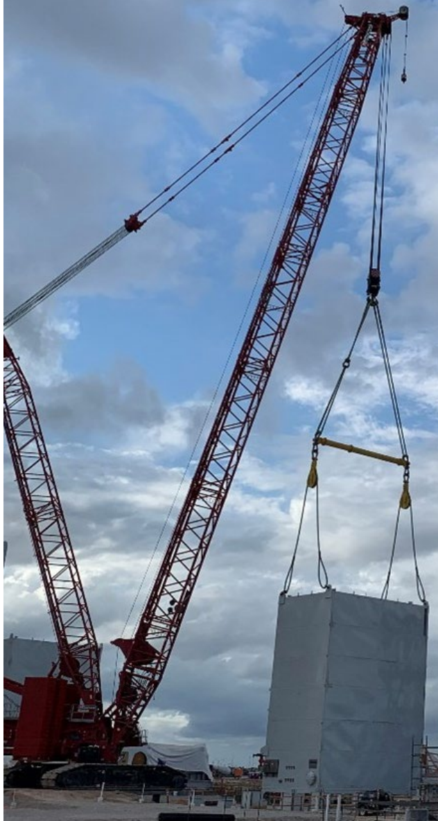
Photo 3: Train 6 Liquefaction Cold Box Set
