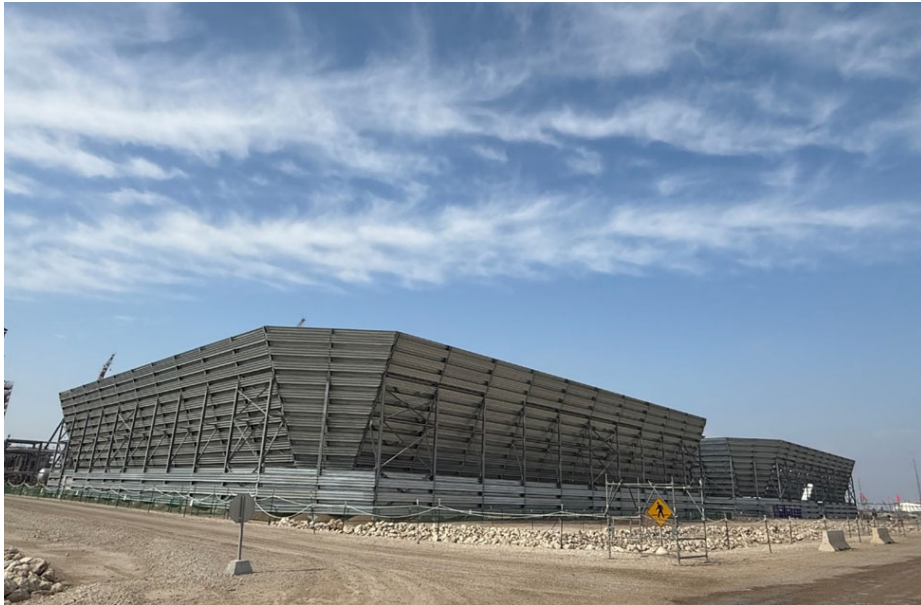
Photo 4: Ground Flares 1 and 2
