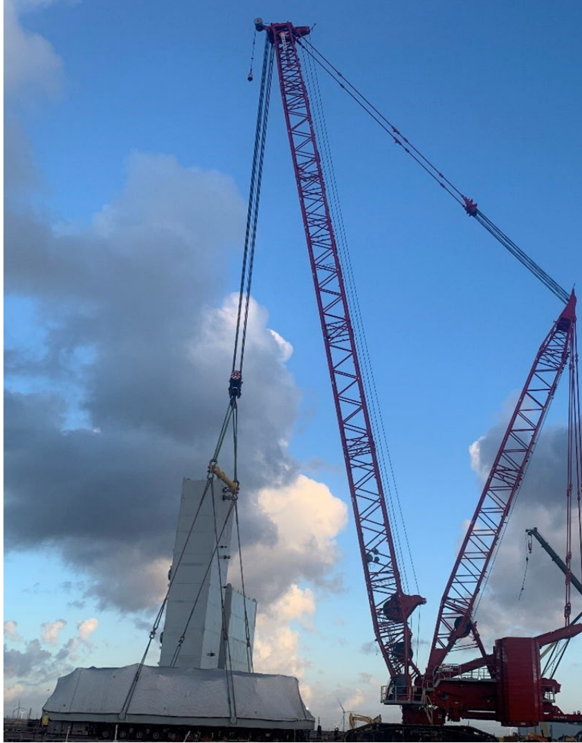
Photo 2: Train 6 Mixed Refrigerant Compressor Set
