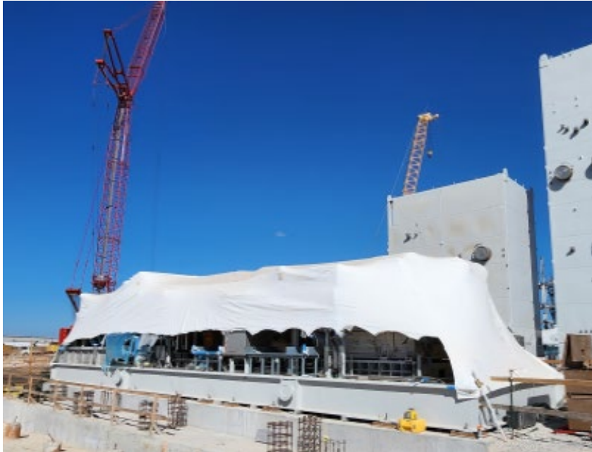
Photo 3: Train 6 Mixed Refrigerant Compressor Set
