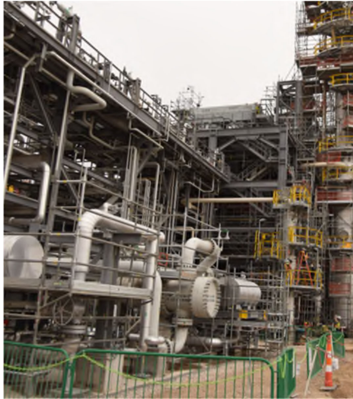
Photo 1: Train 1 Amine Solvent Regeneration Area Startup Isolations
