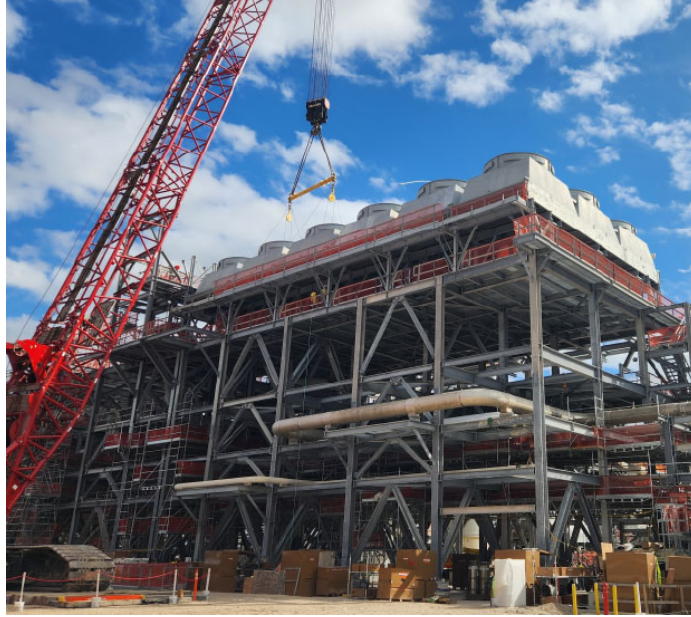
Photo 2: Train 3 Air-Cooled Heat Exchanger Set
