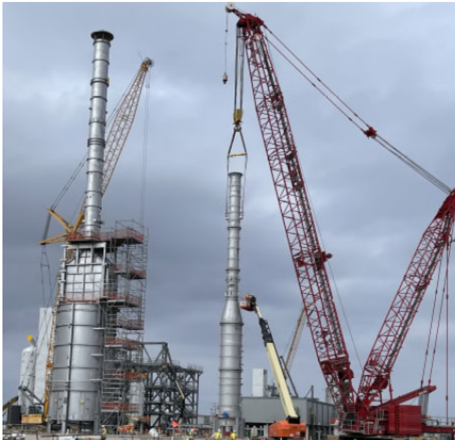
Photo 2: Train 6 Thermal Oxidizer Stack Set
