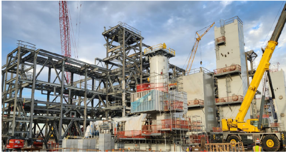
Photo 1: Train 5 Compressor Area Equipment
