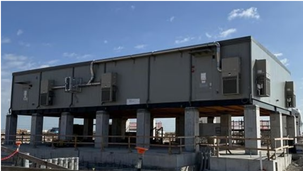
Photo 4: Train 6 Liquefaction Substation Set
