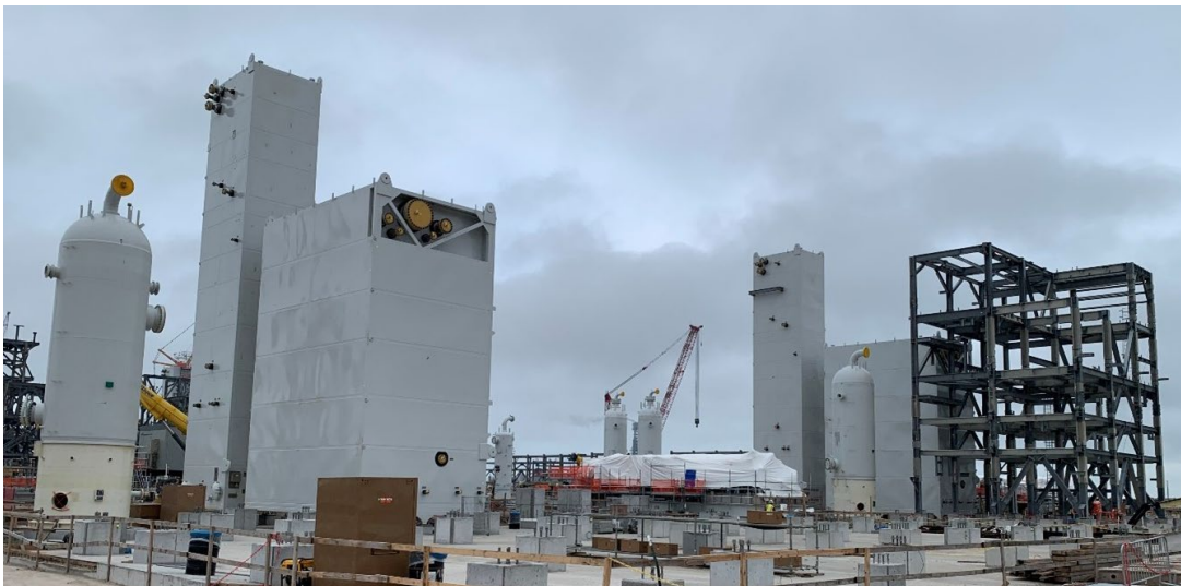
Photo 2: Train 5 Cryo Rack Area
