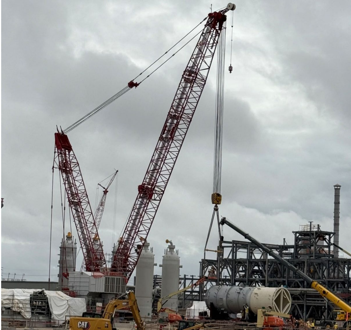
Photo 4: Train 6 Surge Drum
