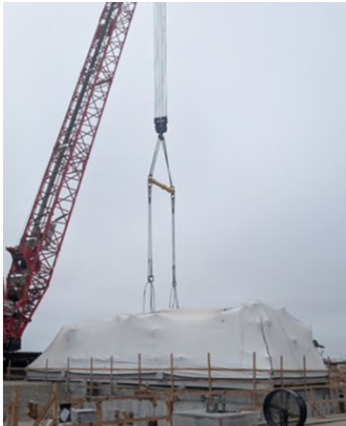
Photo 3: Train 7 Mixed Refrigerant Compressor Set
