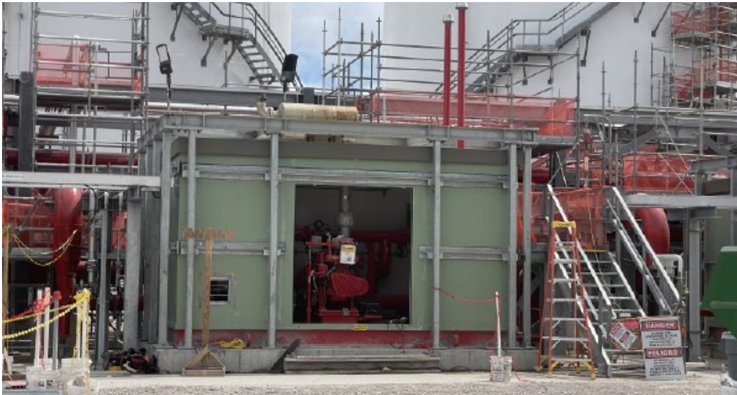
Photo 1: OSBL Diesel Firewater Pumps
