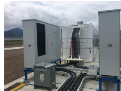
2x1MW GE LV5 Solar inverters
