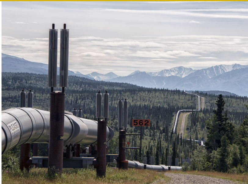
Alaskan oil pipeline, image by Gillfoto, CC-BY-SA-4.0.
