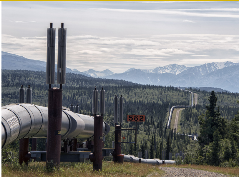
Alaskan oil pipeline, image by Gillfoto, CC-BY-SA-4.0.
