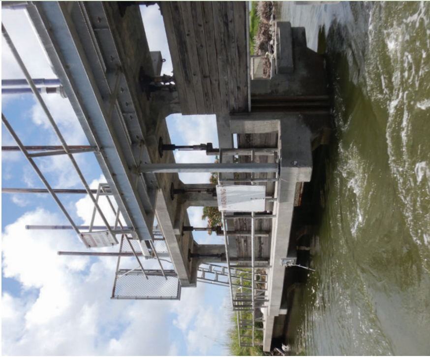
Image: Cameron-Creole Hydrologic Control Structure, 2022 (CPRA)
