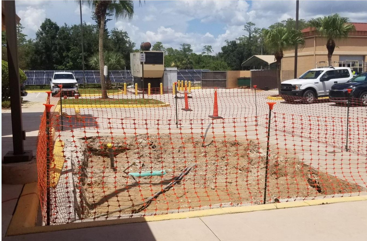
Unmarked sanitary sewer line conflict
