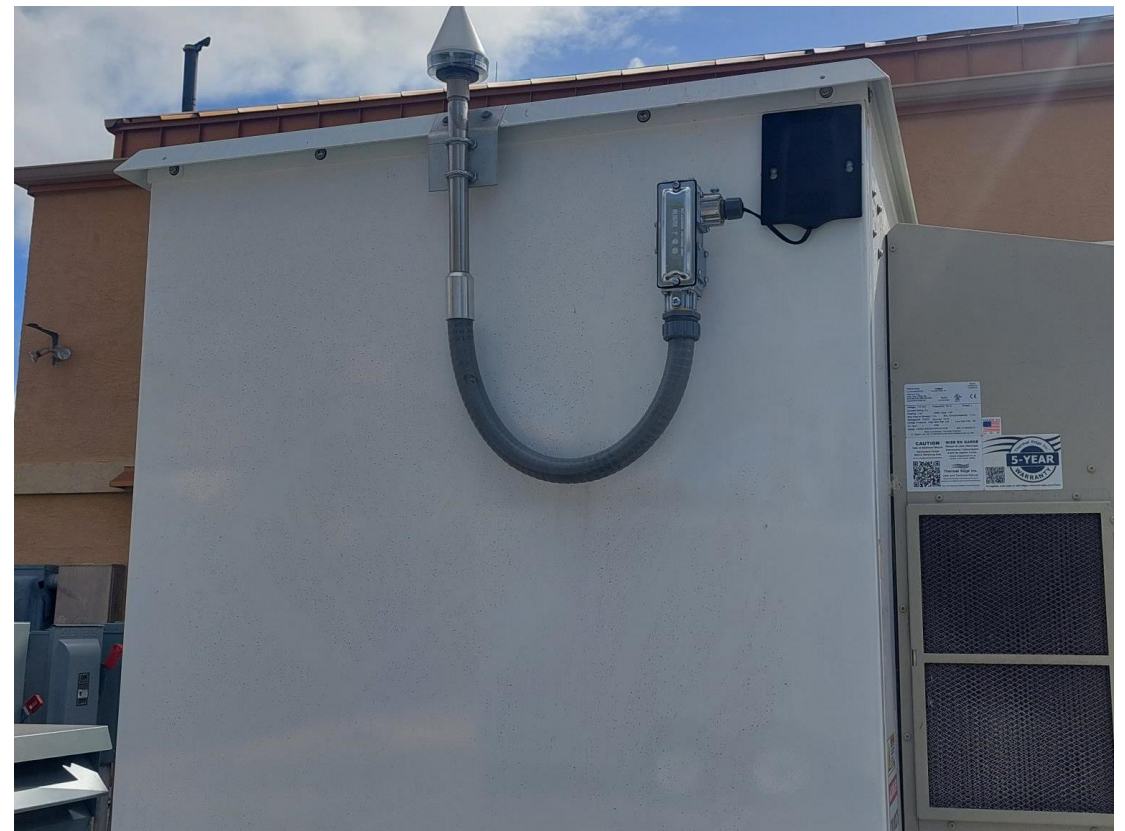
Cellular Modem not transmitting when enclosed in cabinet. Needed antenna.
