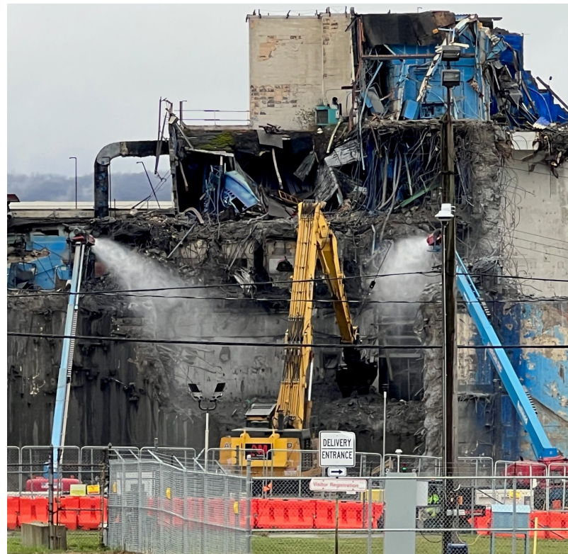
Main Plant Process Building deconstruction of the hot cells, which were used during spent fuel reprocessing operations.
