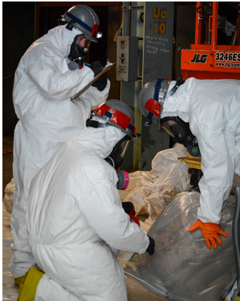
During deactivation workers remove thousands of components from the X-333 building in preparation for future demolition.
