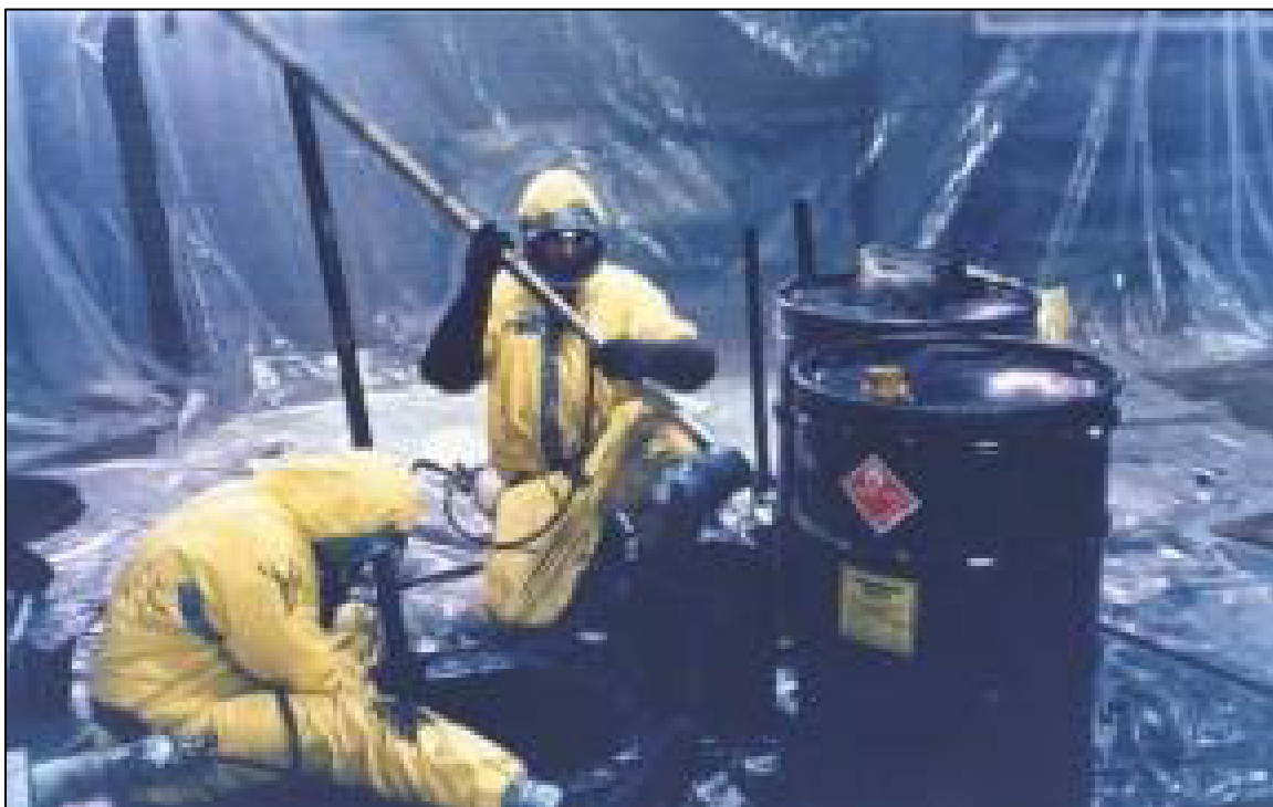
Figure 11-2. Removing Sludge and Placing It in Drums at the Chicago North Site (DOE Digital Archive)
