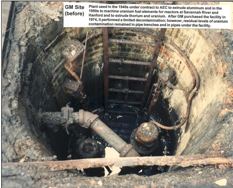
Figure 3-2. Manhole at the Adrian, Michigan, Site Before Remedial Action, December 1974 (DOE Digital Archive)
