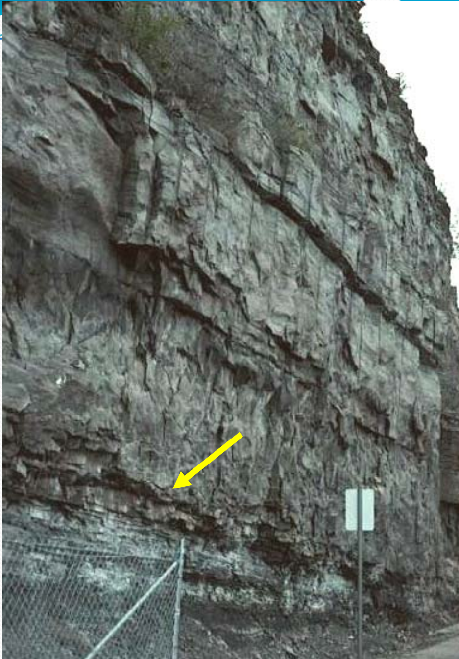
Seepage at the Niagara Gorge
