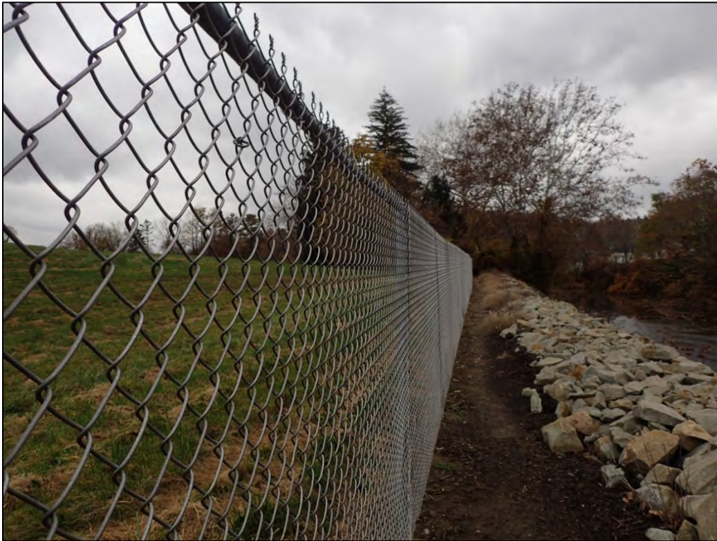
PL-1. Riprap Along Streambank
