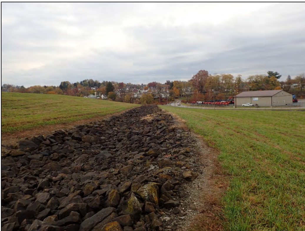
PL-8. Riprap-Armored Diversion Channel
