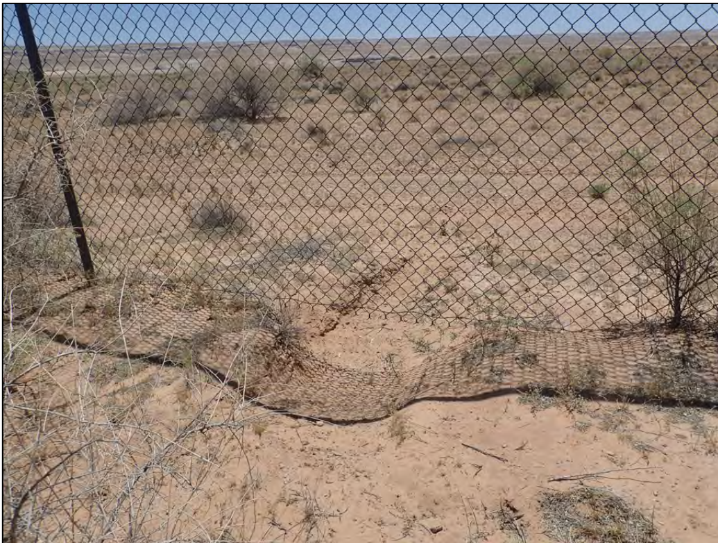
PL-4. Gap Under Perimeter Fence near Perimeter Sign P9
