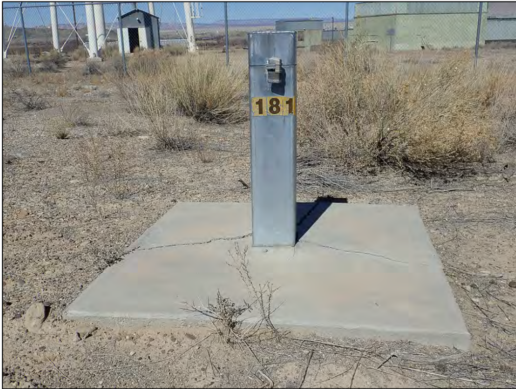
PL-7. Cracked Concrete Around Monitoring Well 0181 (Onsite) and Abandoned Mill Buildings (Offsite)
