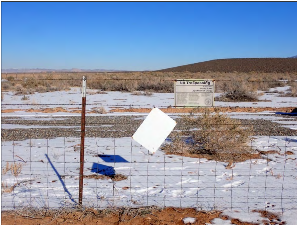
PL-4. Partially Detached Perimeter Fence Sign
