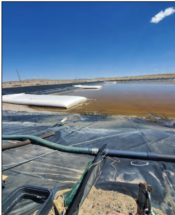
PL-10. Evaporation Pond with hydrologic barriers deployed to mitigate seepage
