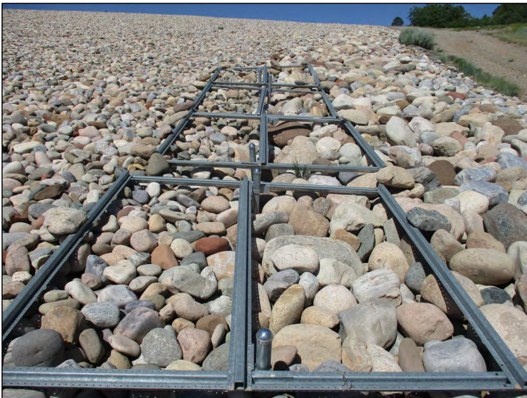
PL-6. Depression on North Toe of Disposal Cell Before Repair
