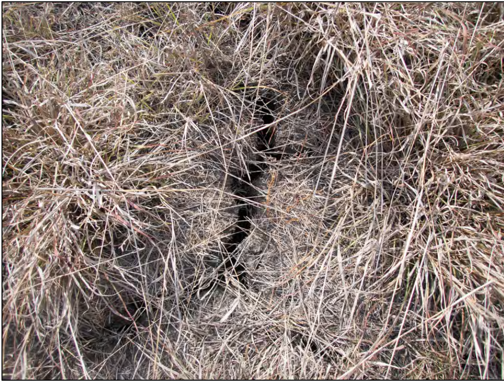
PL-7. Soil Desiccation Cracks on Top Slope of Disposal Cell
