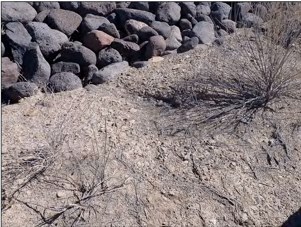
PL-10. Soil Erosion Along Southwest Side Apron (Onsite)
