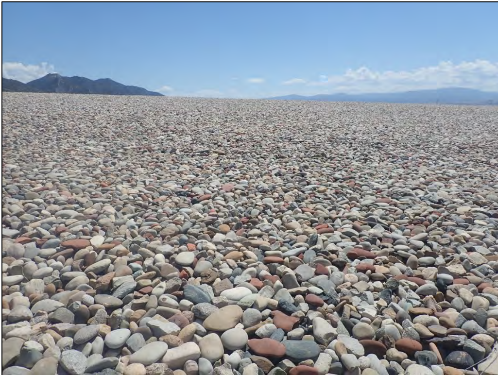
PL-8. Potential Depression on Edge of Disposal Cell
