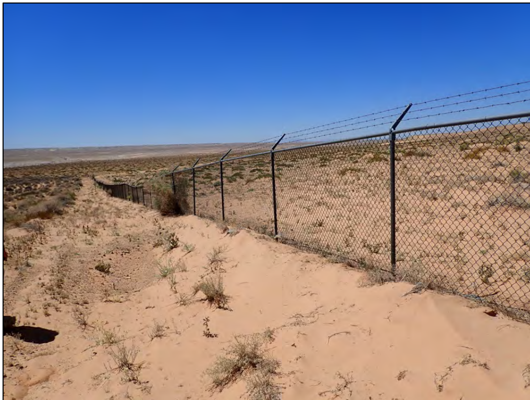
PL-2. West Perimeter Fence with Sand Deposition
