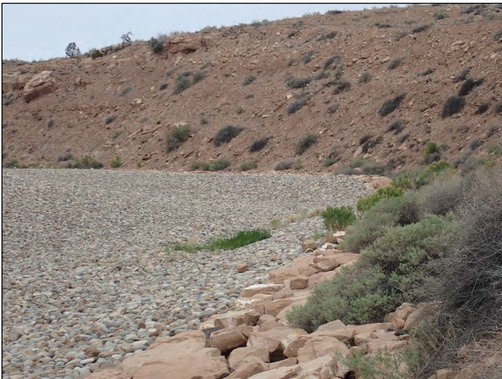
PL-6. Vegetation Growing in Accumulated Sediment Downslope from Culvert Break
