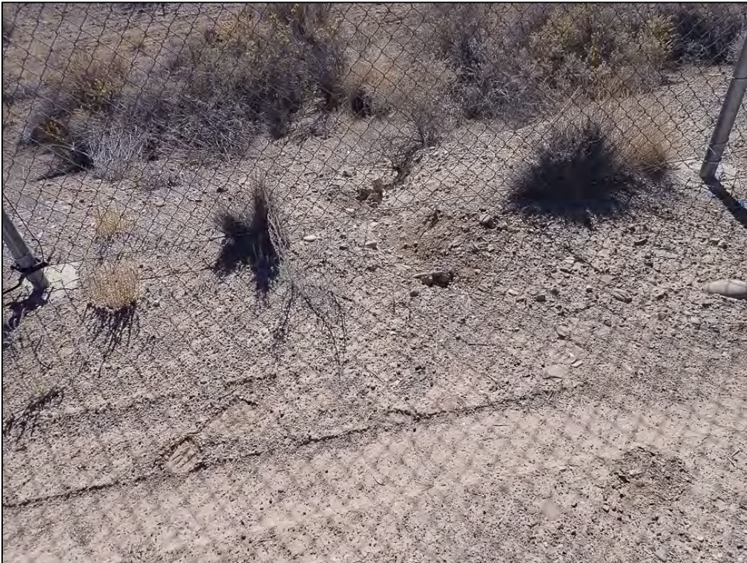
PL-12. Soil Erosion Along Southeast Side Chainlink Security Fence
