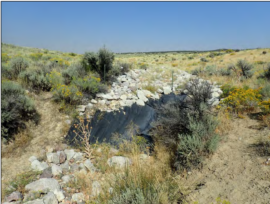
PL-12. Exposed Geofabric in Swale No. 1
