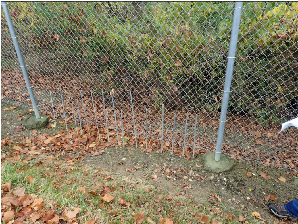
PL-2. Slats in Fence at Erosion Area
