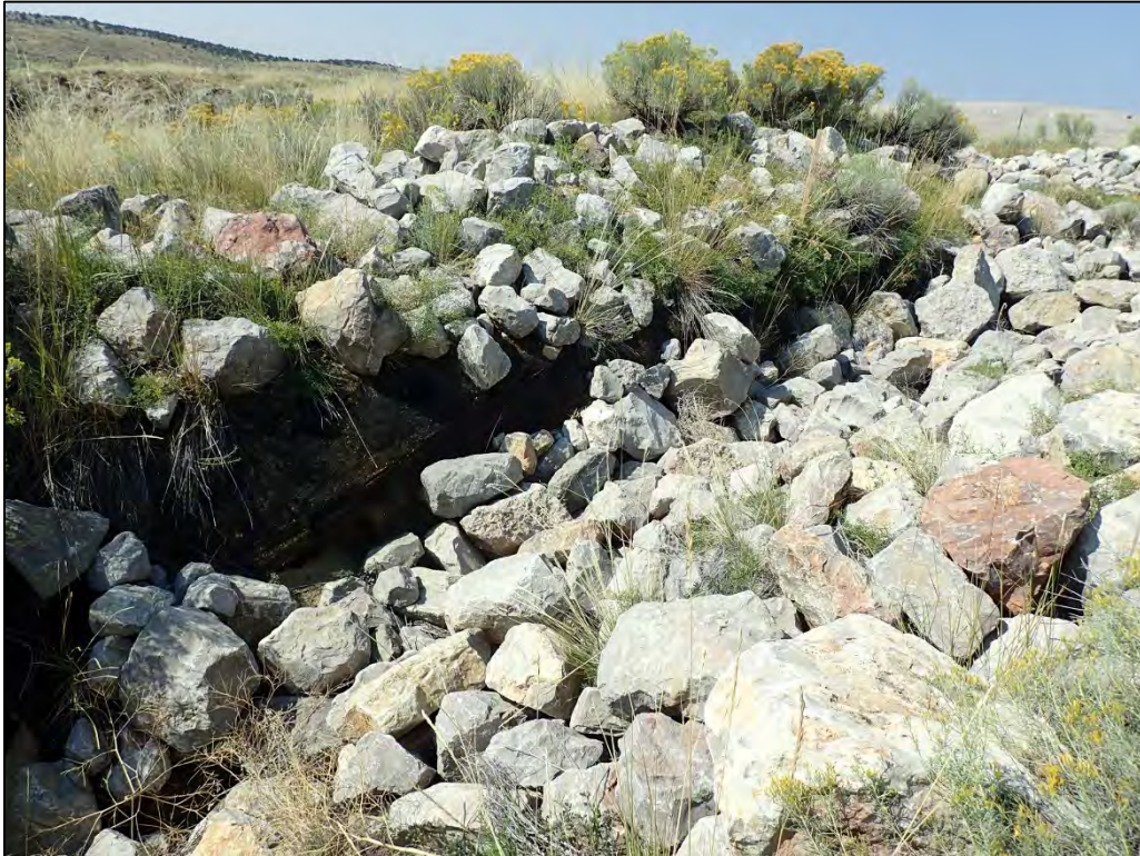
PL-13. Exposed Geofabric in Swale No. 2
