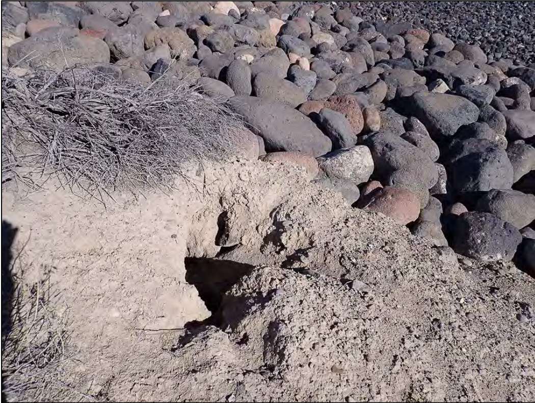
PL-11. Possible Soil Piping near South Corner of Disposal Cell
