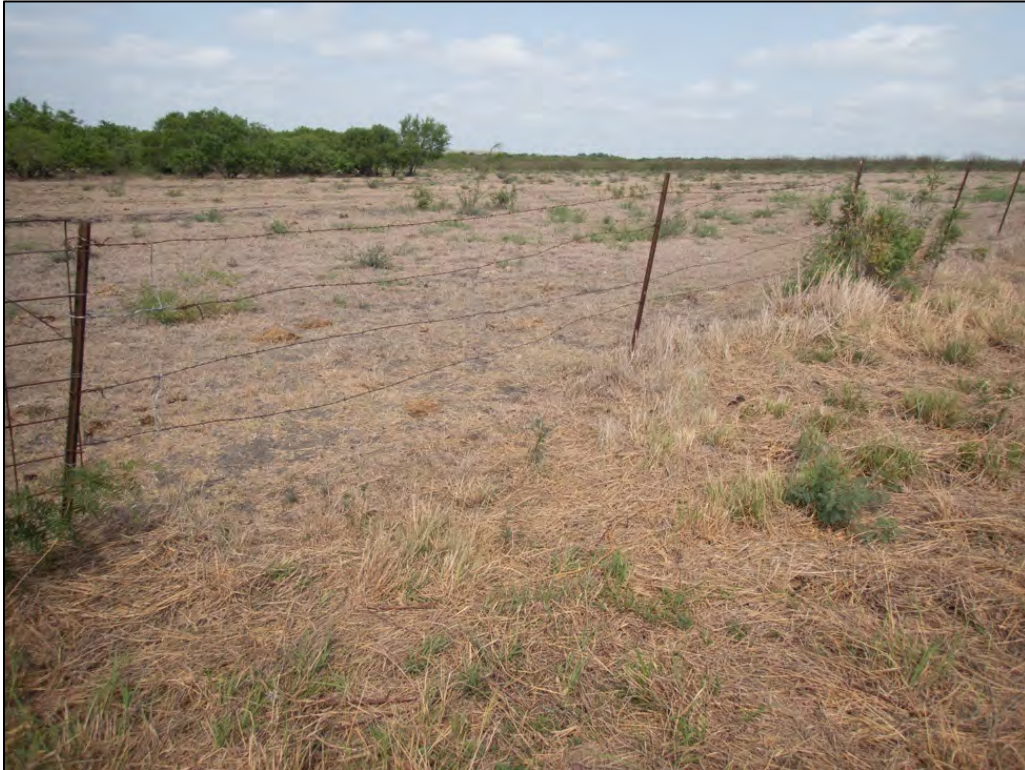
PL-1. Rusted and Damaged Fence Line
