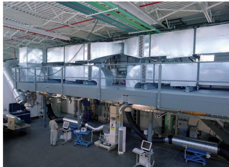
NREL's HVAC Laboratory
