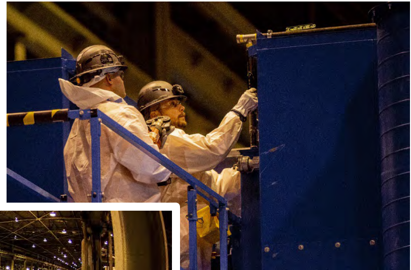
Compressed air piping for dust collection system
