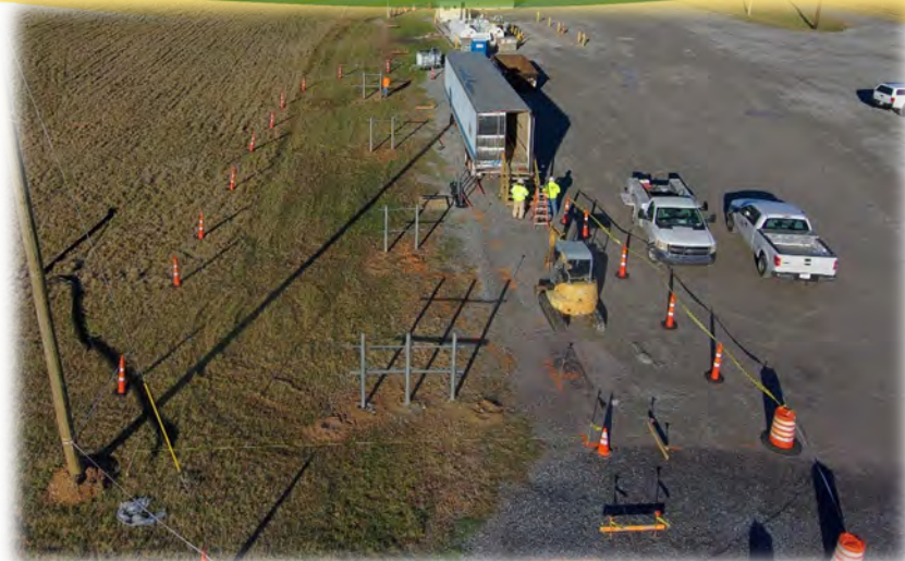
Near C-752-B Fuel Station
