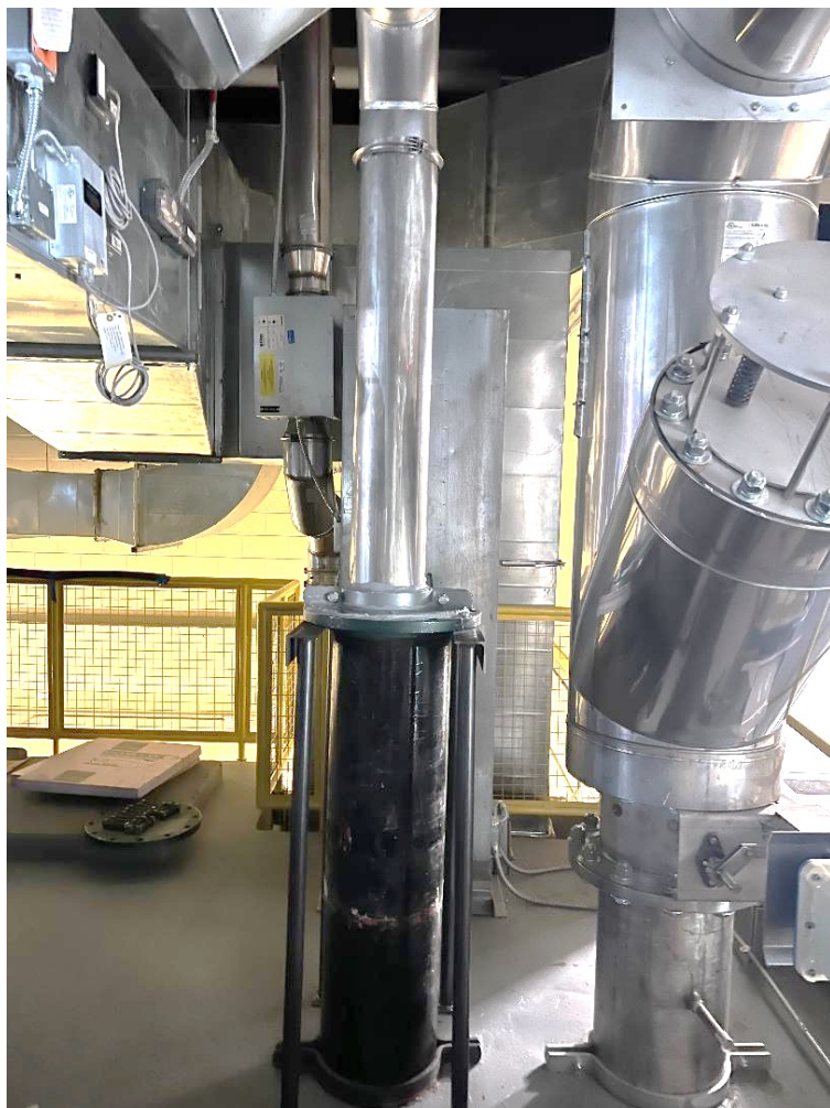
Dilution tunnel designed and installed at UA
